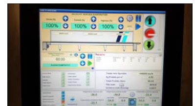
Digital Control Panel
