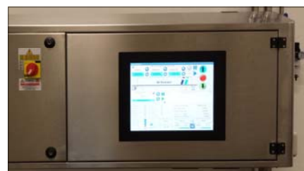
Digital Control Panel
